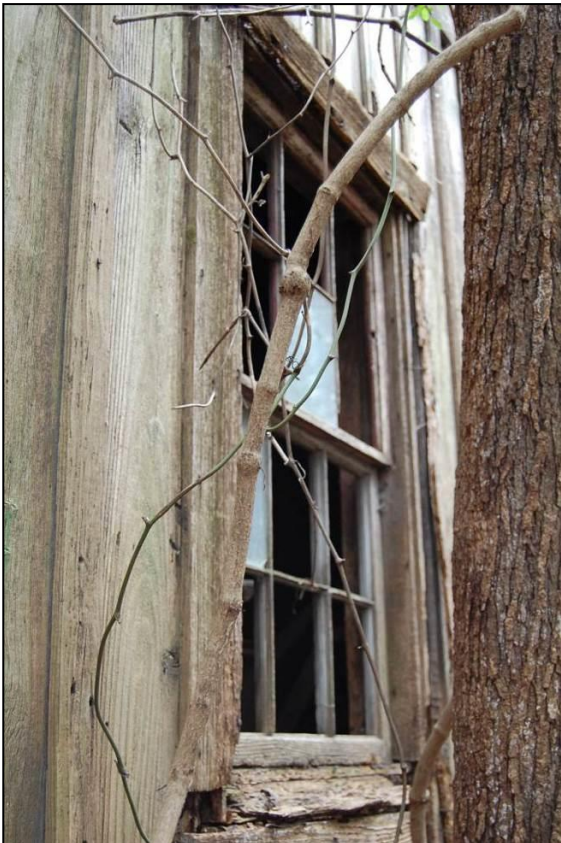
Figure 33. Board-and-batten walls and six-over-sash window at far right of southwest front elevation of bunkhouse
