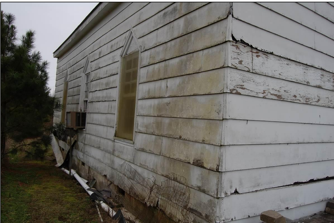
Figure 100. Jericho A.M.E. Zion Church Fellowship Hall, long north and gabled west elevations
