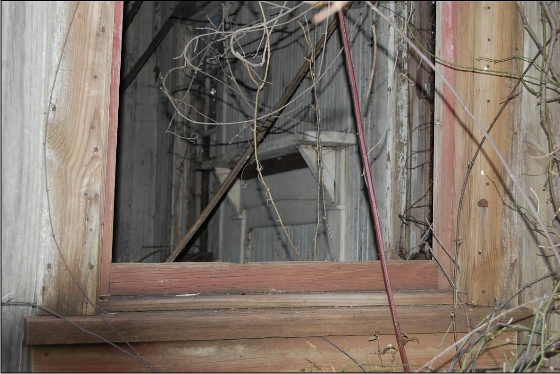
Figure 195. Graingers Railroad Section House, mantel and tongue-and-groove wall boards in front block's east room
