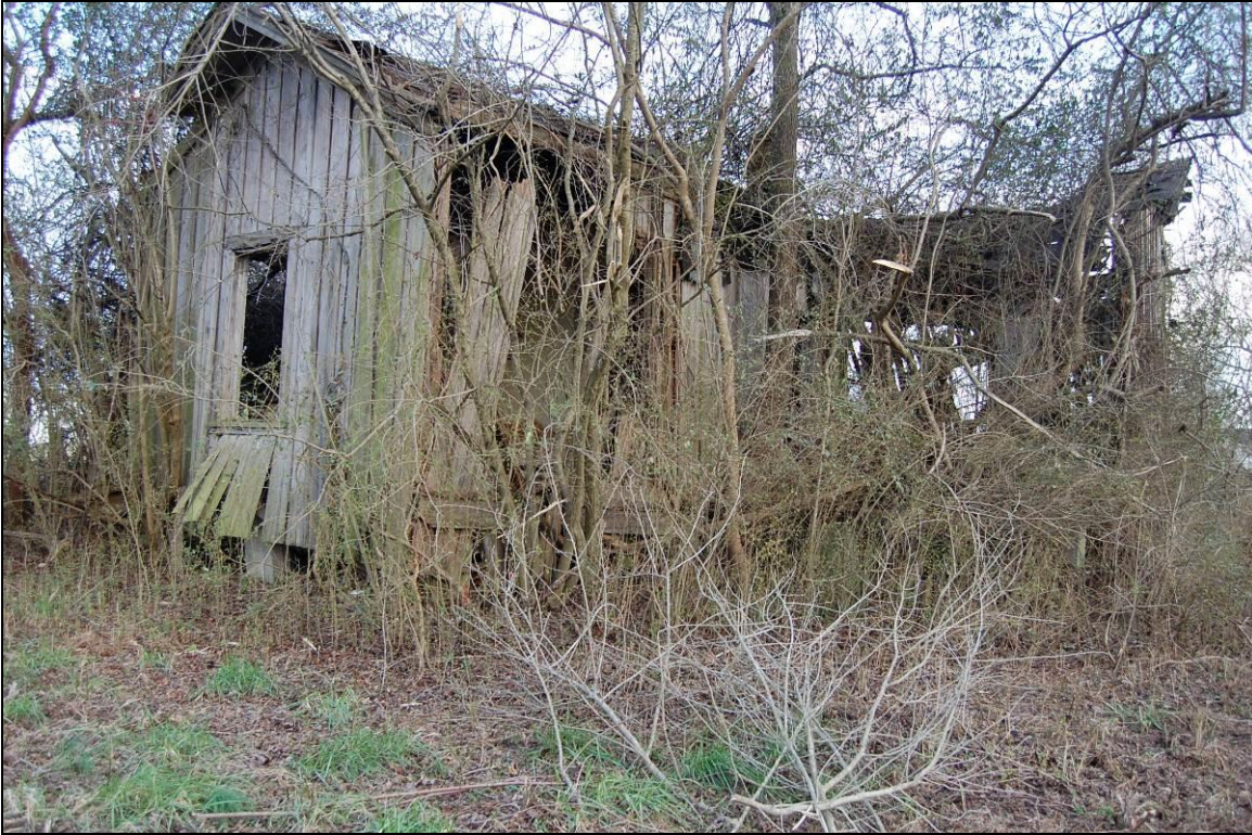
Figure 197. Graingers Railroad Section House, looking southeast at collapsed walls of front block at right and ell at left
