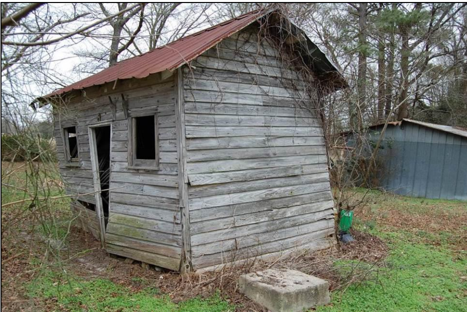
Figure 40. Toolshed, southwest side and northwest front elevations; northwest side elevation of farm equipment shed at right
