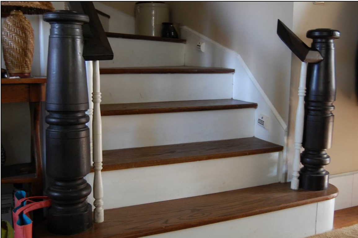
Figure 143. Altered stair in front block of house with original or early newel posts
