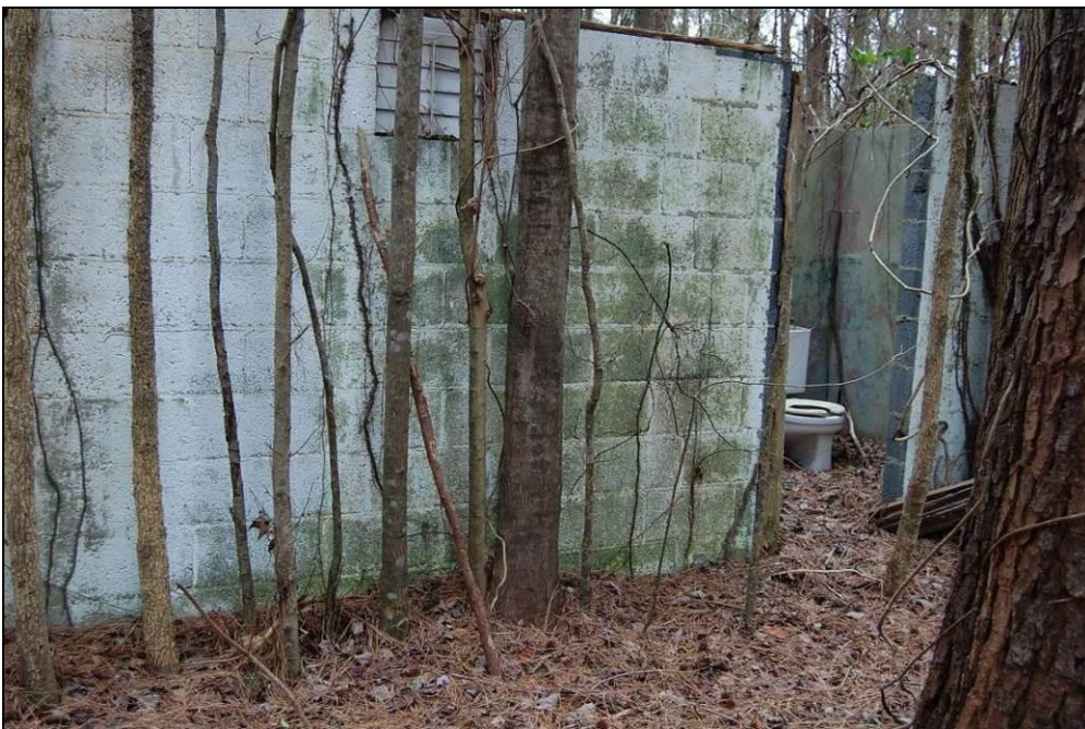
Figure 112. North side elevation of rear section of projection building, which held bathrooms
