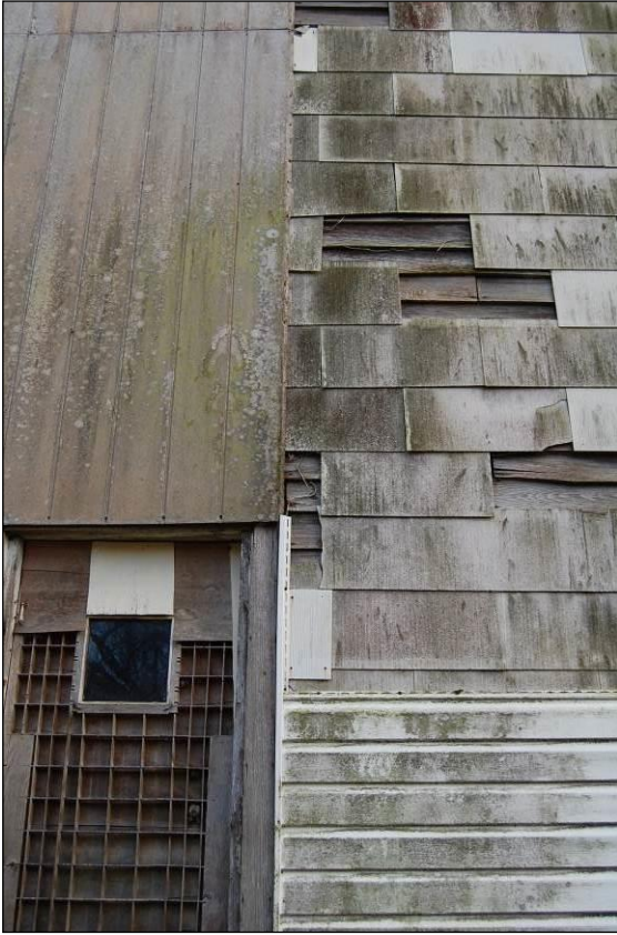
Figure 189. Northwest rear elevation detail of door and composition board, vinyl, asbestos, and weatherboard siding
